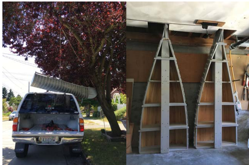
A block and tackle was used to hoist the form off the truck. Holes cut into the ceiling allowed the forms to stand upright.
